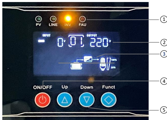
Figure 13 elements control panel
